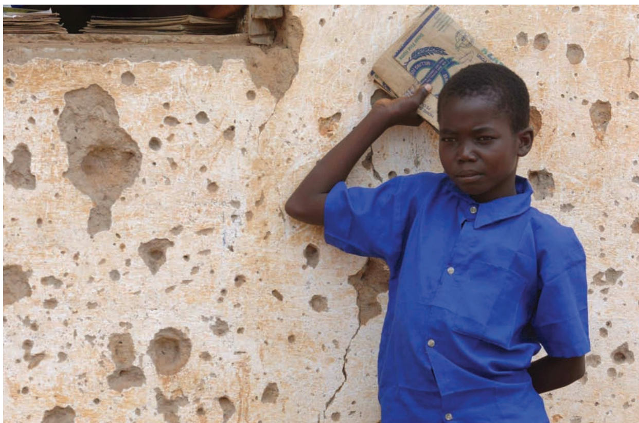
Thousands of bullet holes riddle the facade of this school and remind returnees in Yei of their painful past, Sudan 2005. © UNHCR M. Pearson.
