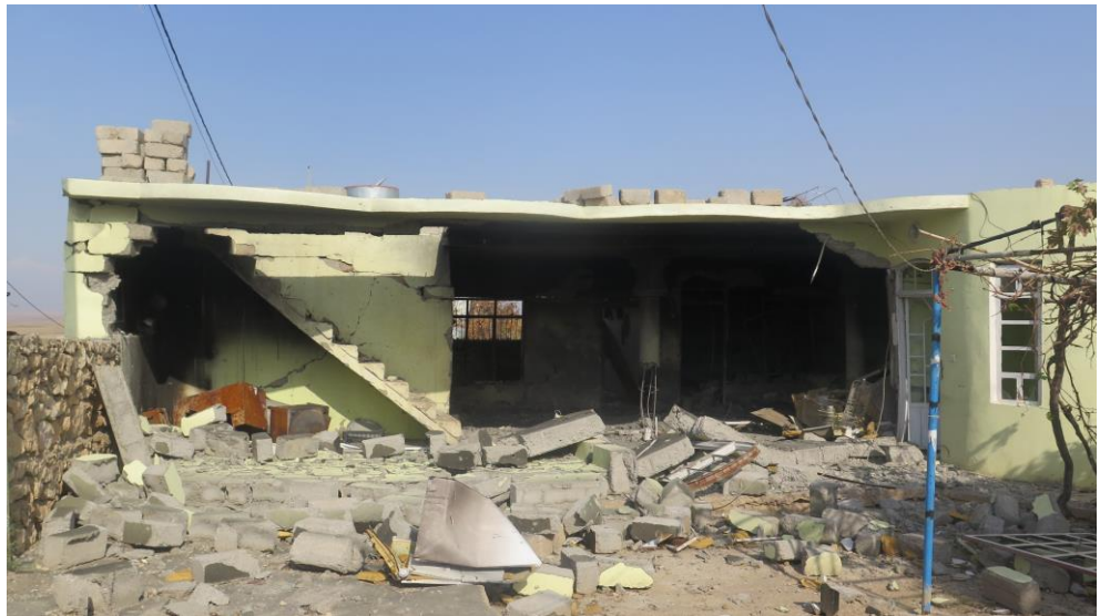
Destroyed house in Barzanke © Amnesty International
